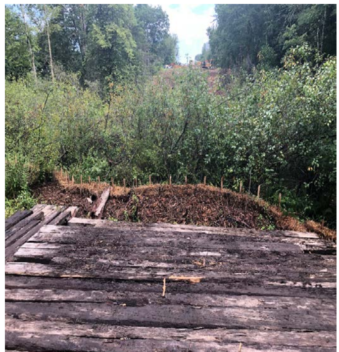
Fig 20: Siltation controls installed between Str. 28 work pad and wetland DW49. Viewing north. (8-14-19).
