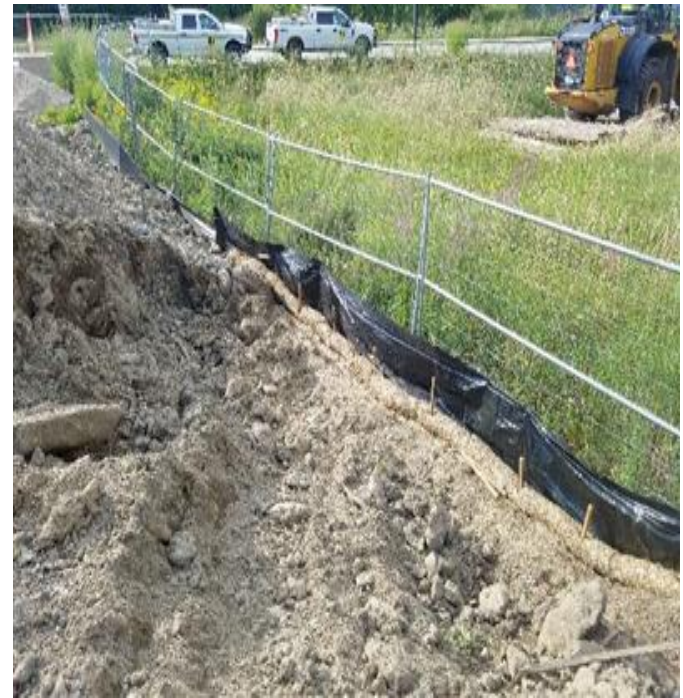
Fig 8: Perimeter and silt fence repairs made in Waterworks Rd laydown yard. Viewing west. (8-12-19).
