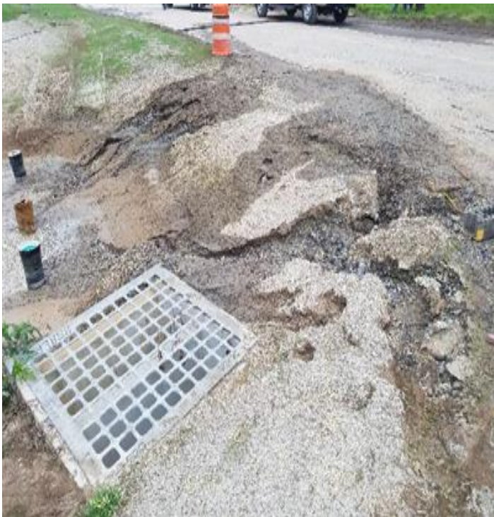
Fig 11: Erosion rills observed on slopes of the rain garden cont. Viewing north. (8-13-19).
