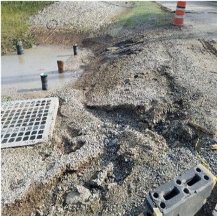
Fig 9: Erosion rills observed on slopes of the rain garden. Viewing north. Viewing south. (8-12-19).
